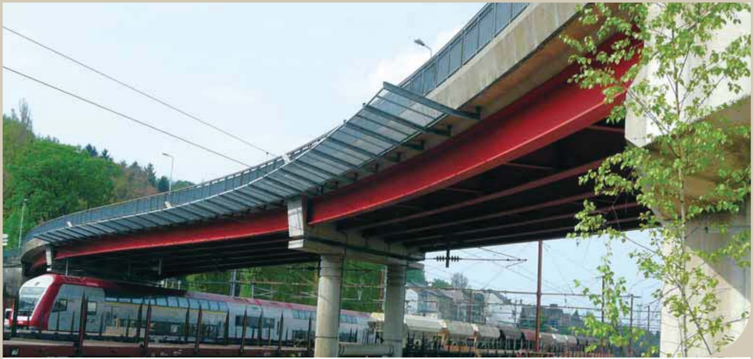
Roadbridge in Differdingen, Luxembourg – Bridge with a strong bending over the weak axis (see erection of two main girders on page 7).
