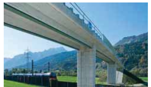
The Vigaun bridge made of PreCoBeams with three spans of 26.15 m and a slenderness ratio of 1/23.
