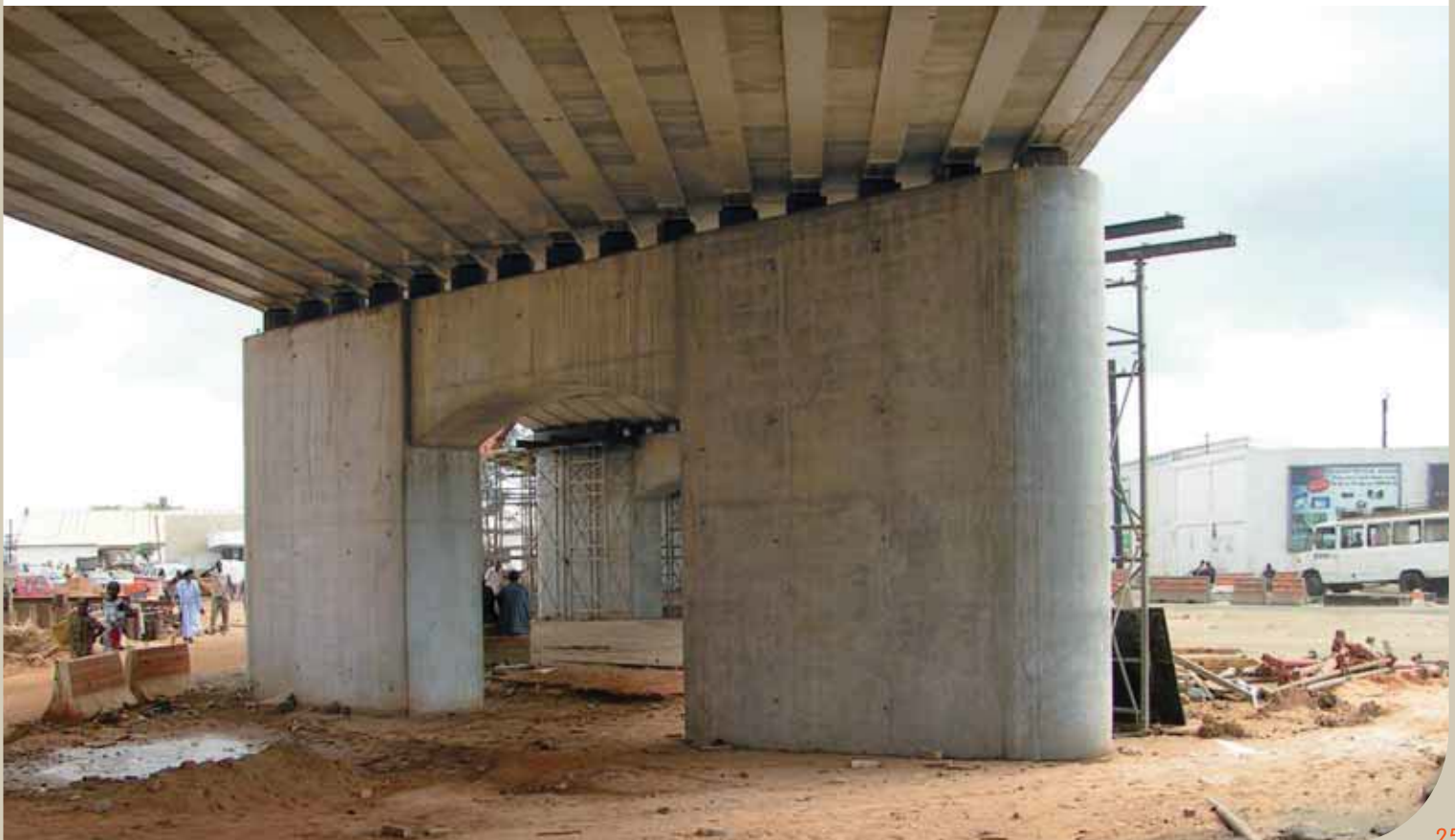
Pont de Cyrnos in Senegal - Bottom view on the filler beam deck and support.
