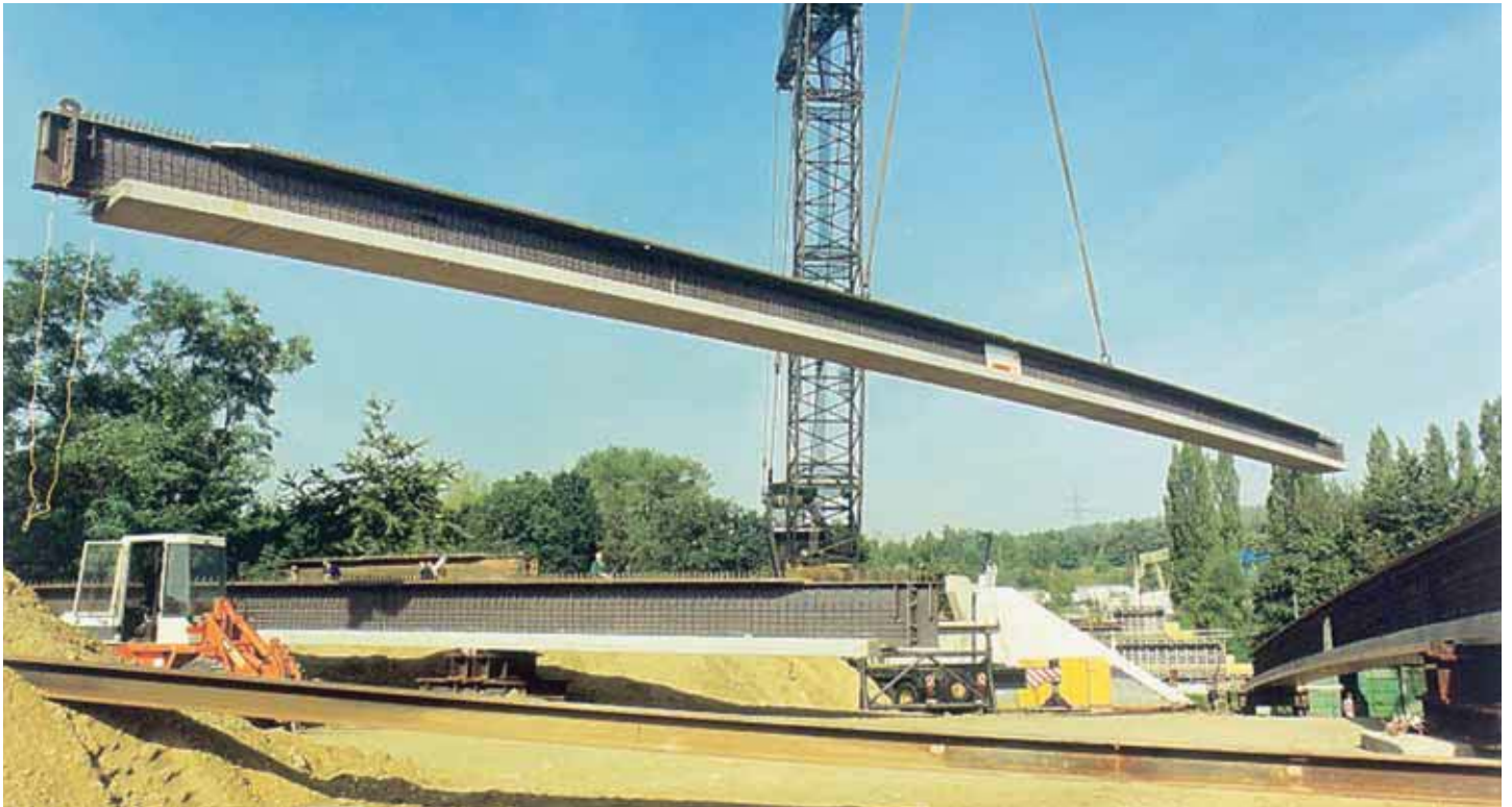
Single span bridge in Kerpen Horrem, Germany - 41.25 m long HE 1000 A beams used for prestressed composite girders of "Preflex" type.
