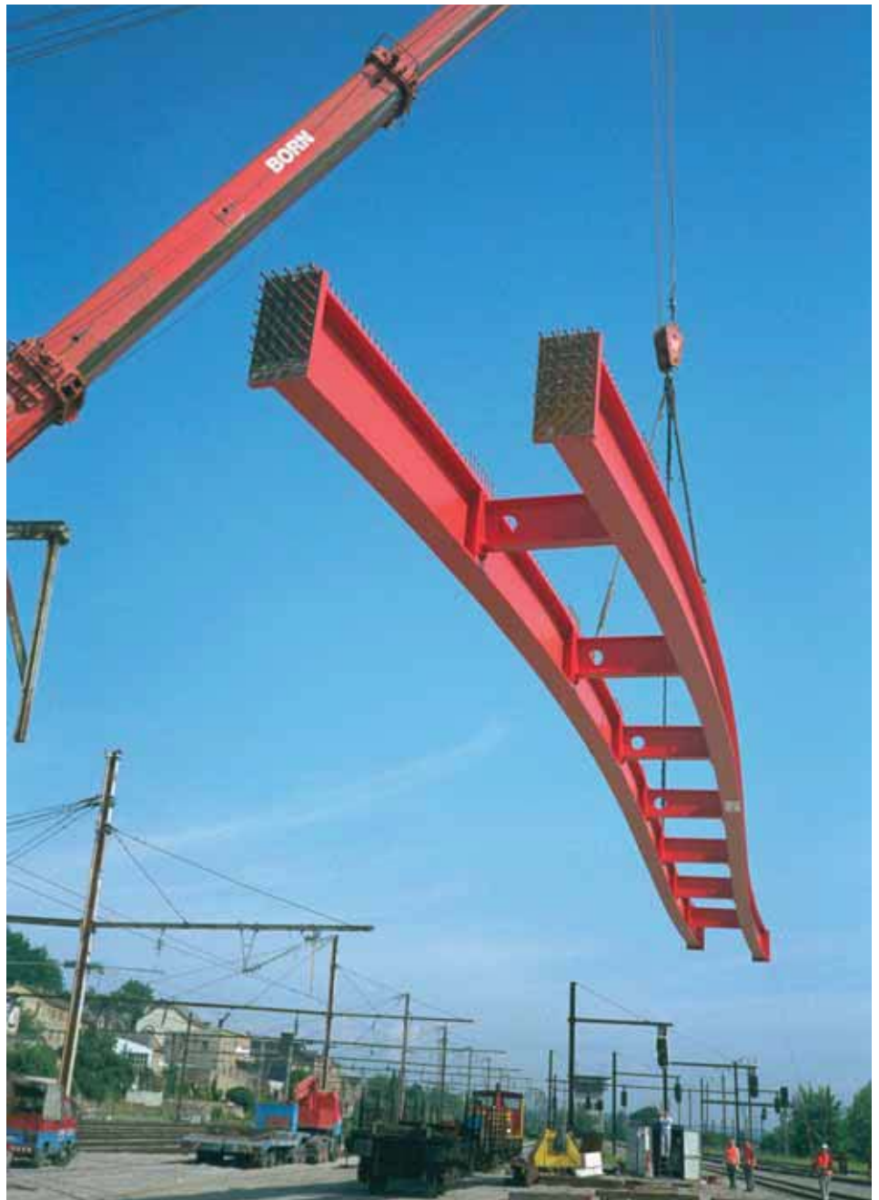
Road bridge in Differdingen, Luxembourg – Erection of two main girders of a composite bridge by crane. The rolled girders are curved along both cross-sectional axes in order to adapt them to the geometry of the road.
