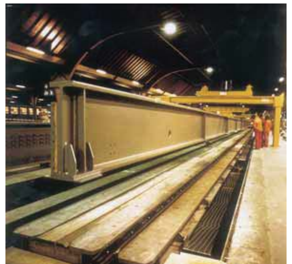
Renovation of the platform in the main station in Zürich - The new 5-span decks for ballasted track are of half through girder type with rolled beams and a reinforced concrete slab supported on lower flanges. Available time and space dictated the erection procedure. The 69 m long beams were lifted into position with portal cranes.
