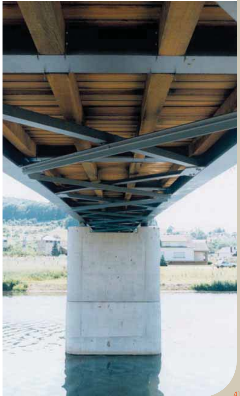
Bottom view on the stiffening elements of the bridge in Steinheim, Luxembourg
