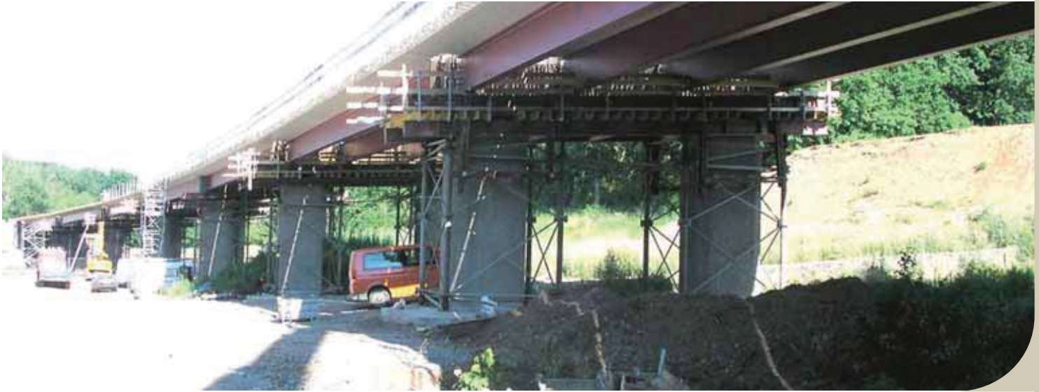
The Horlofftalbridge in Hungen (Germany) with eight spans constructed in 2006. For five spans partially prefabricated concrete beams with heavy rolled beams in S460 have been used.
