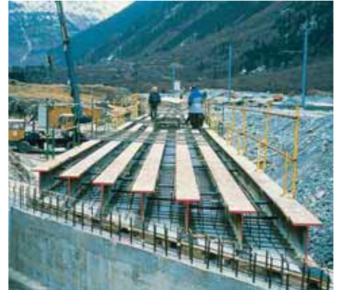
Construction of a filler beam railway bridge as part of the Puymorens road tunnel link between France and Spain.
