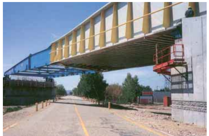
A half-through girder deck during launching. It carries the new Mediterranean High Speed Railway Line which was opened to traffic in 2002. The exposed flanges of the transverse filler beams can be seen at the bottom side. The blue coloured part is the launching nose.
