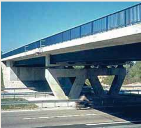
Road bridge in Bremgarten, Germany - With concrete cross beams and indirect support.
