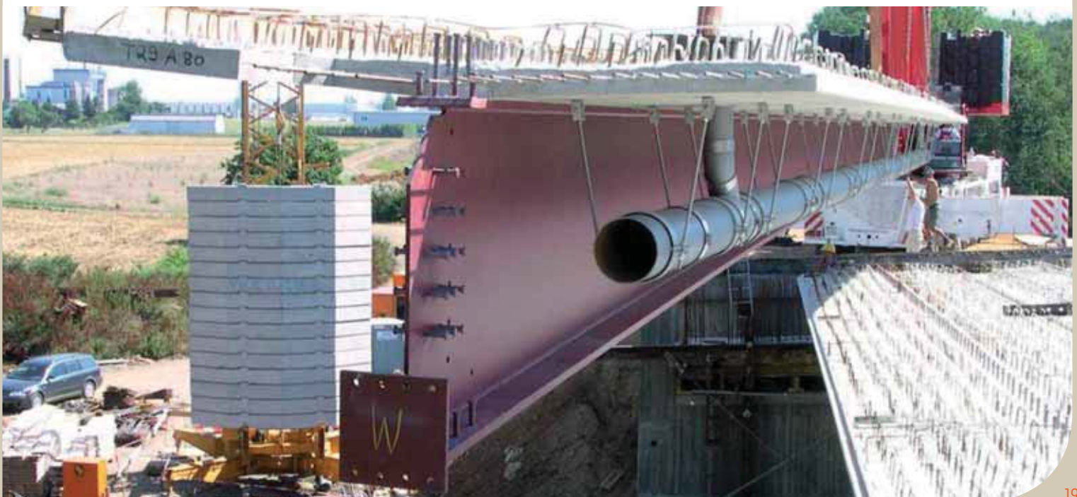
The Horlofftalbridge in Hungen, Germany - Lifting in of a partially prefabricated beam.
