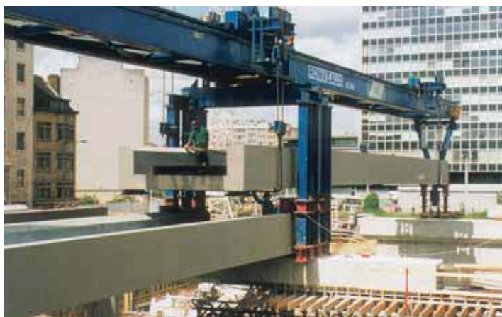
Extension of the Brussels - South Station for the Eurostar trains - A launching gantry is used for fast erection of prefabricated prestressed composite decks.
