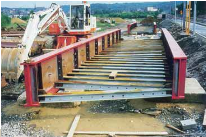
Railway bridge over the Emile Mark street in Differdange, Luxembourg - The replacement of an old deck with direct track fastening by a ballasted track bridge required a structural system with minimized construction depth. A half-through girder deck solved the problem. The picture shows the assembled steel framework before concreting.
