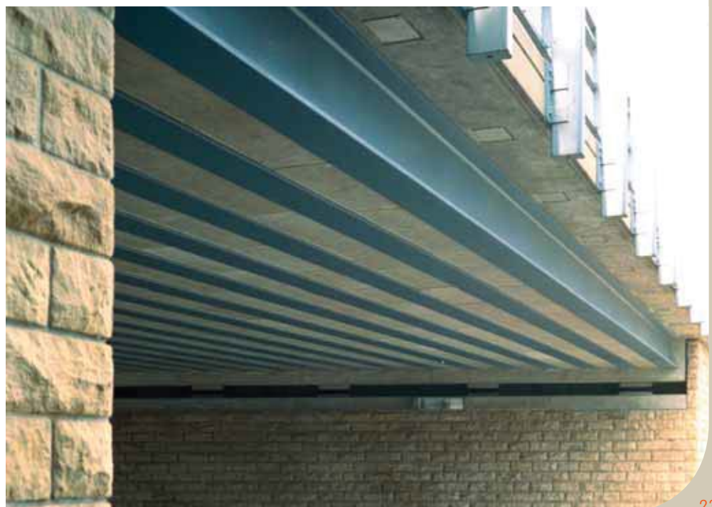
Lower side of a filler beam deck - Only the bottom flanges of beams are visible.
