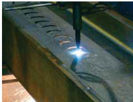
Oxycutting of a rolled beam (HD 400x421 in S460) with the shark fin shape for the PreCoBeam bridge at Vigaun, Austria.
