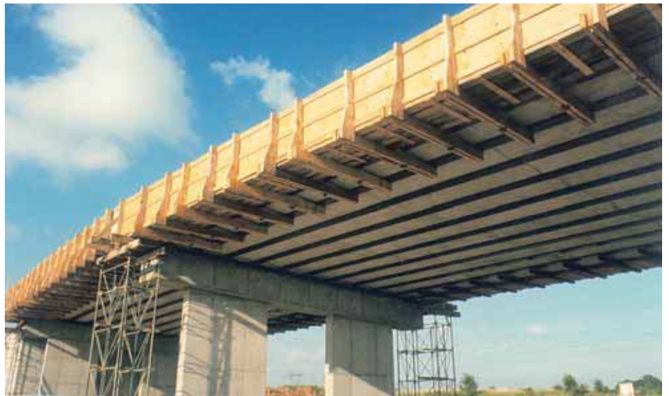
Construction of an overbridge of A104 motorway, France – Falsework is not required. Disruption of motorway traffic is minimal.
