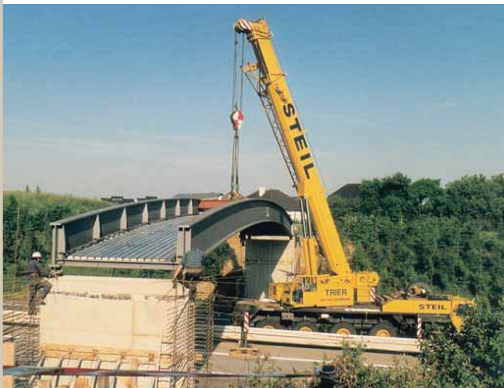
Erection of half-through type structure - Pre-assembled framework including permanent steel shuttering is lifted into position by crane.
