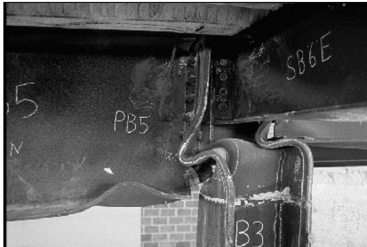
Figure 2.7 Squashed column head following the test
