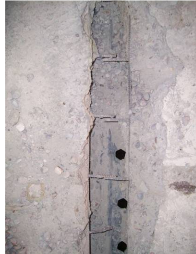
(b) State of the reinforcement joint at the location of the crack after cooling
