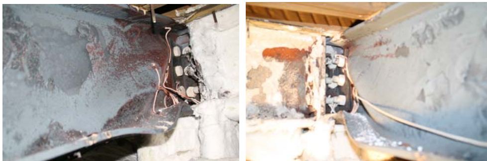
Figure 7.39 Local buckling of unprotected secondary beams connected to
