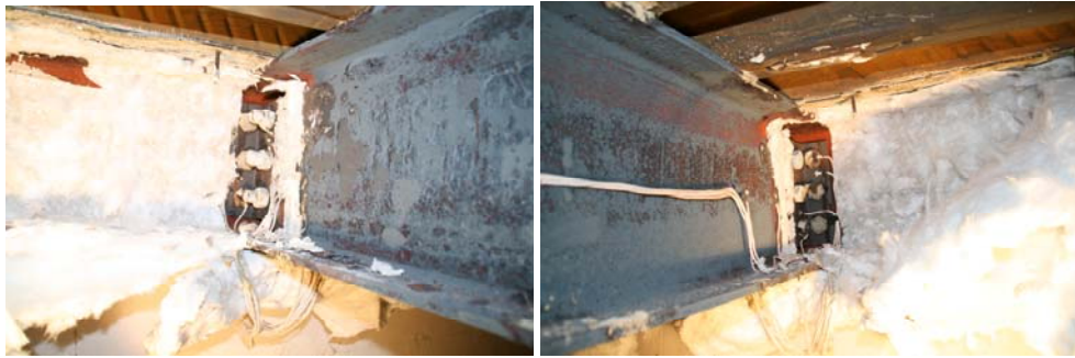
Figure 7.40 No local buckling of unprotected secondary beams connected to main beams
