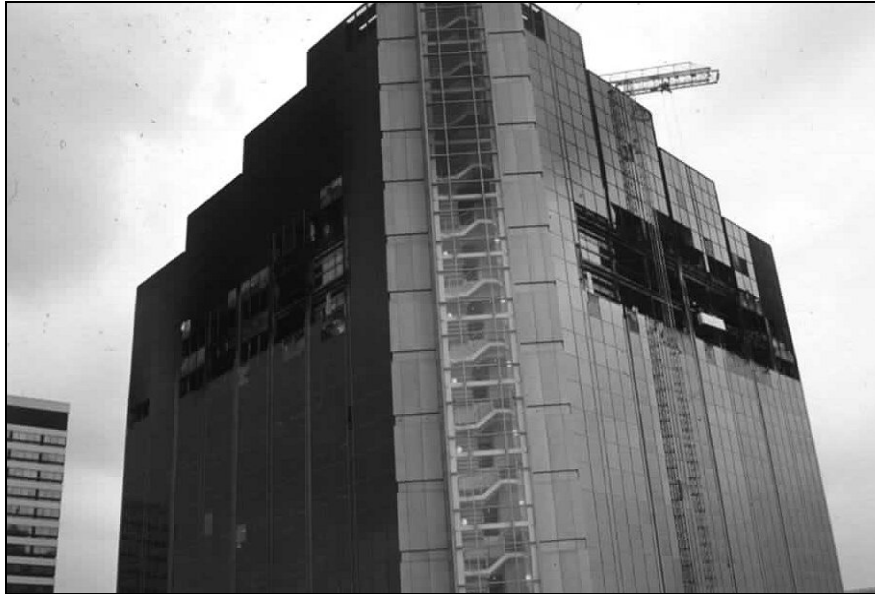
Figure 4.3 Churchill Plaza, Basingstoke following the fire
