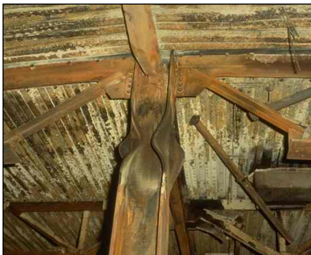
Figure 4.1 Buckled column and deformed beams at Broadgate
