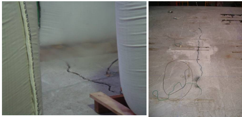
(a) State of the cracking at central part of the floor
