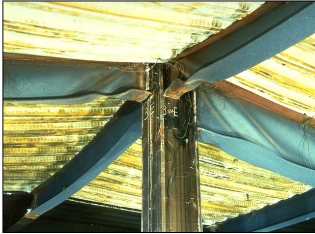
Figure 2.20 Column head showing buckled beams
