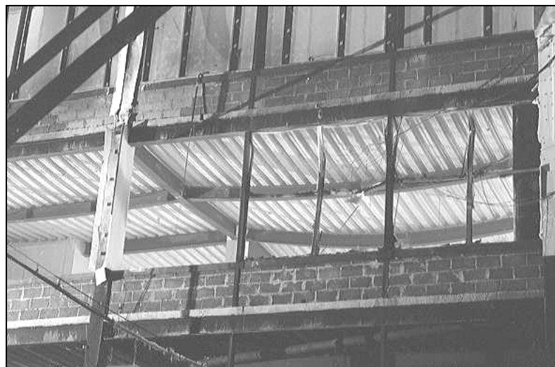
Figure 2.14 Deformed structure during fire
