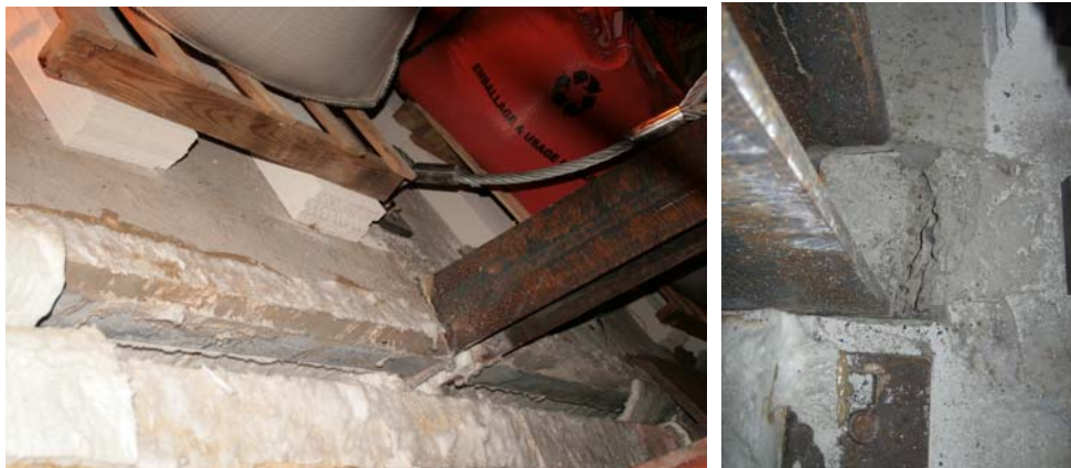
Figure 7.42 Cracking of concrete around central columns
