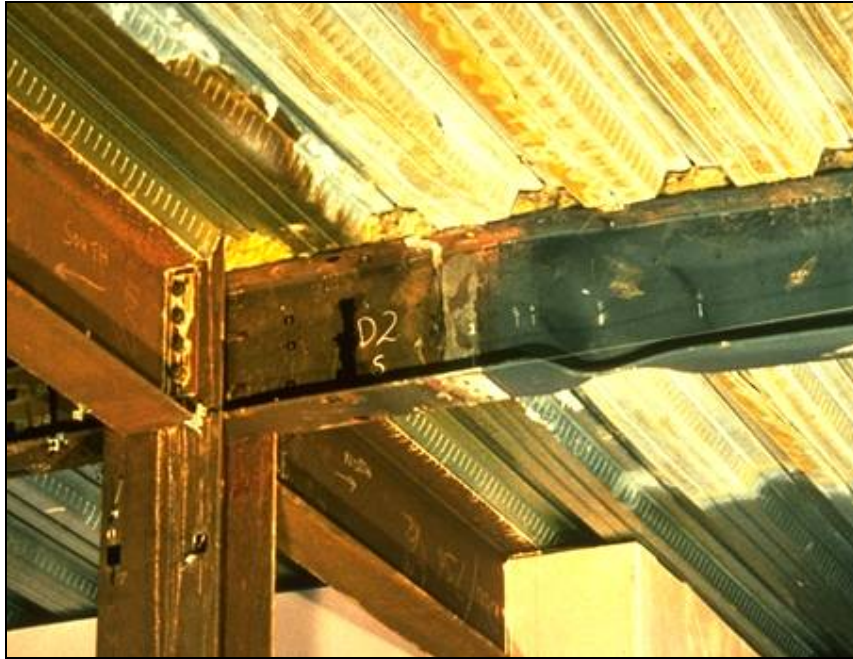
Figure 2.5 Flange buckling in restrained beam
